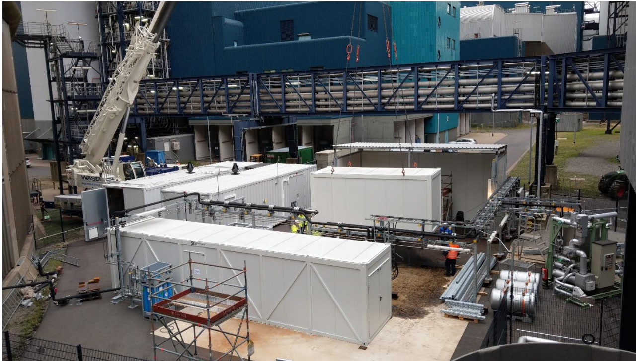
CO 2 capture plant
